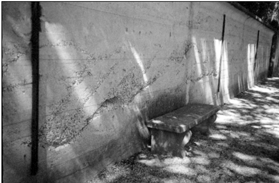
2001 – The rough texture of the concrete walls is an inherent characteristic of their construction, but when losses have increased to a point where they threaten the structural stability of the wall, they must be repaired.
