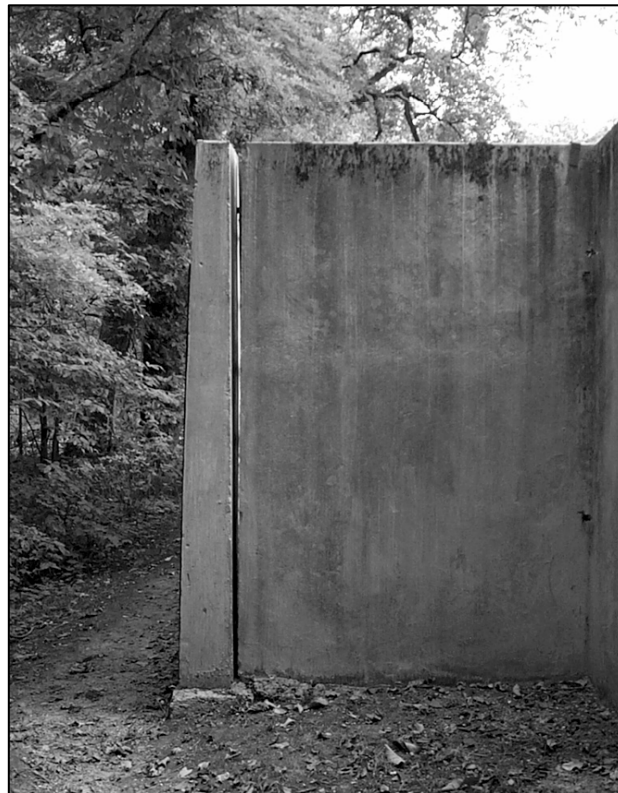
2001 – Some sections of the Sunken Garden wall, such as this area where two sections have separated, require structural stabilization. There are also issues associated with surface treatment and minor losses.
