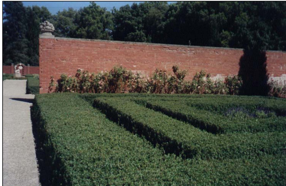
2001 – This view towards the west wall shows the spalling of the wall and the paucity of plantings. The single arborvitae is a post-1946 addition.
