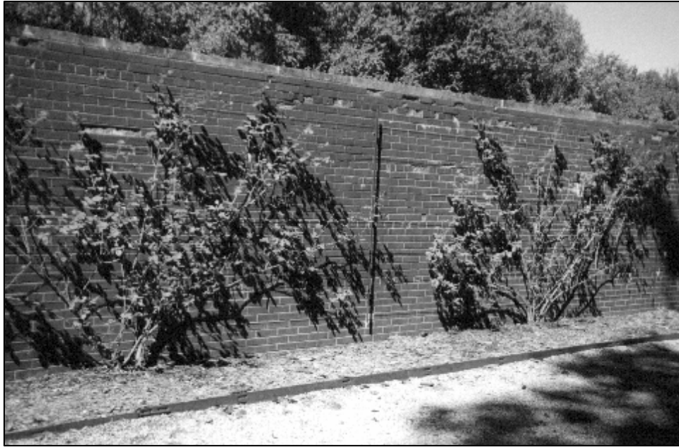
2001 – The brick walls surrounding the Brick Wall Garden (seen here from the Square Parterre Garden) must be repaired prior to any rehabilitation of plantings. The spalling evident in this photo may be due to problems with an improper capstone.
