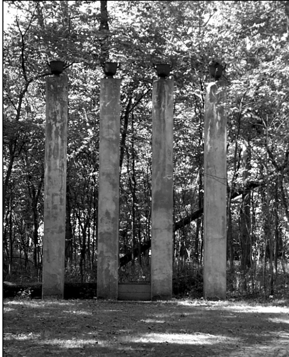
2001 – Pylons associated with the outlying spaces of the Centaur indicate serious deterioration, including evidence of recent losses. This hazardous condition should be rectified as soon as possible
